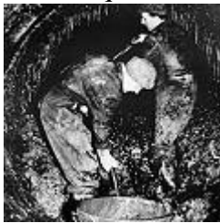
Clearing hundreds of tonnes of mussels from the blocked intake culverts, Marchwood Power Station.
